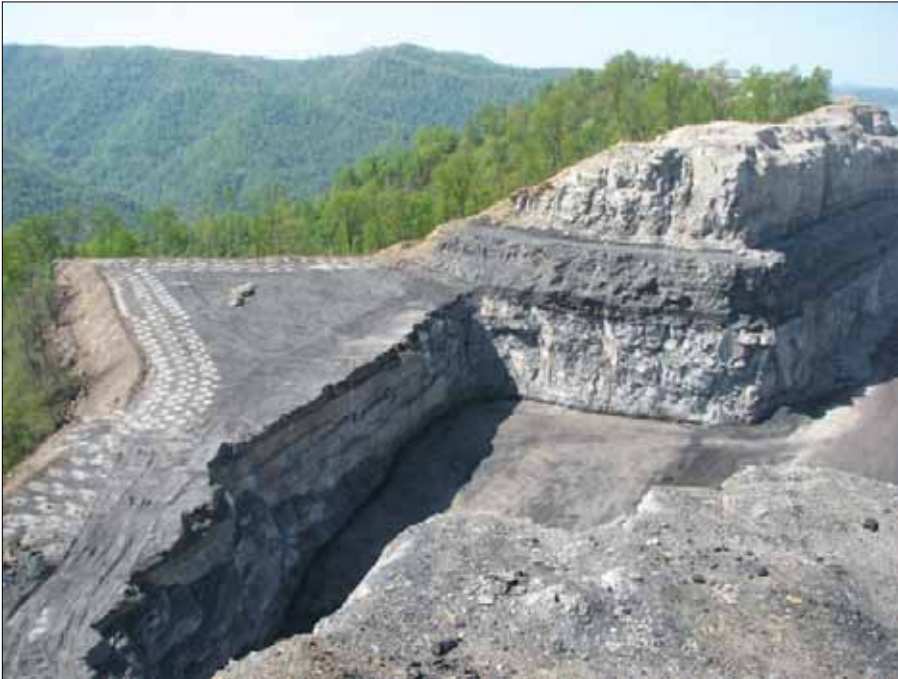
Getting ready for another summertime blast - the three lines of white splotches in this photo are bore holes, packed with hundreds of pounds of explosives to rip away yet more of Kayford Mountain.
