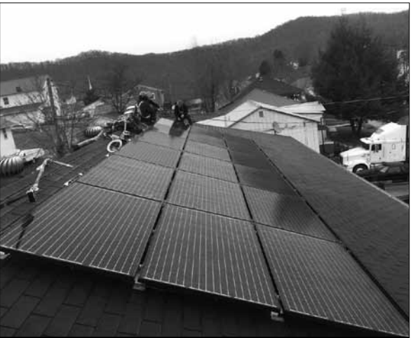
Solar panels on Coalfield Development’s building in Wayne, WV.
